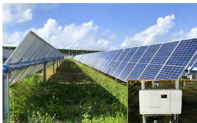
Vitoria Project, Brazil 2.5MW
