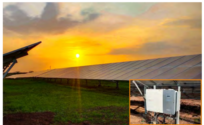
Grow Solar Project, India 10MW
