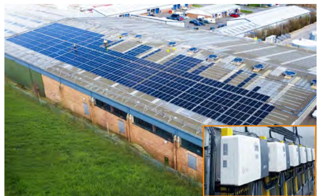
Faerch Plast Project, UK 2MW
