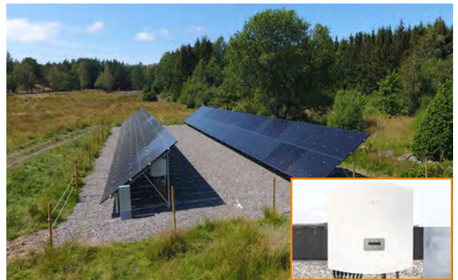
Västra Götaland, Sweden 43.3kW
