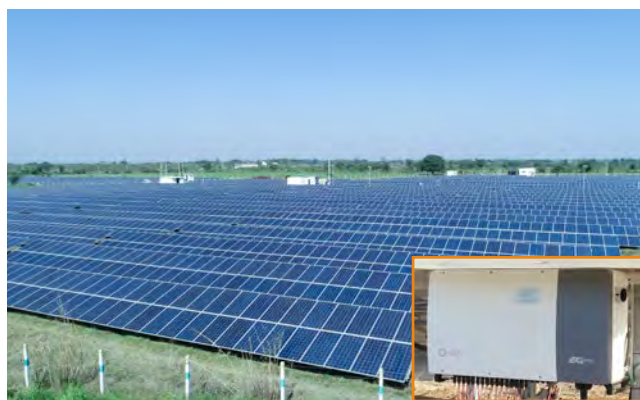
Soleos Energy Project, India 2MW
