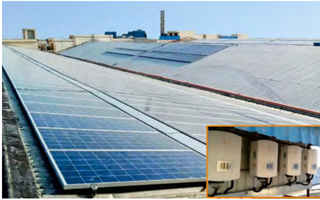
RSWM, India 3.6MW
