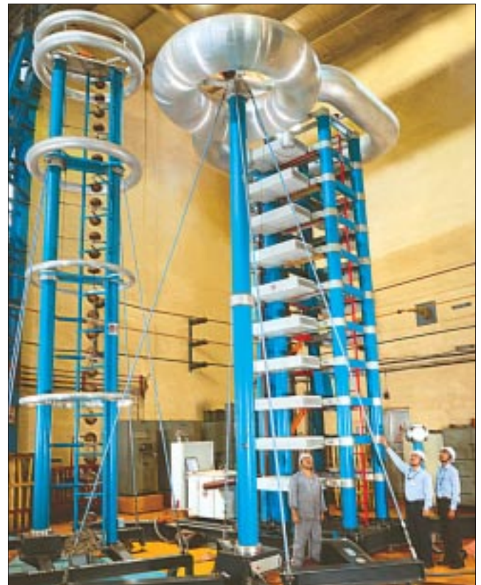
Impulse Generator - 2000kVp
