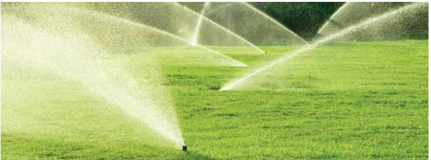
Automatic garden sprinkling system
