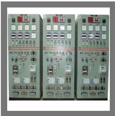
Control and Relay Panel with BCU
