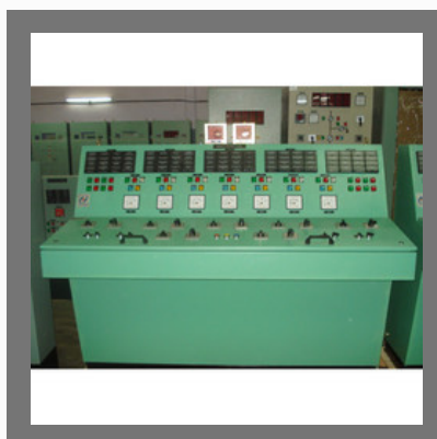
Control Desk Panel
