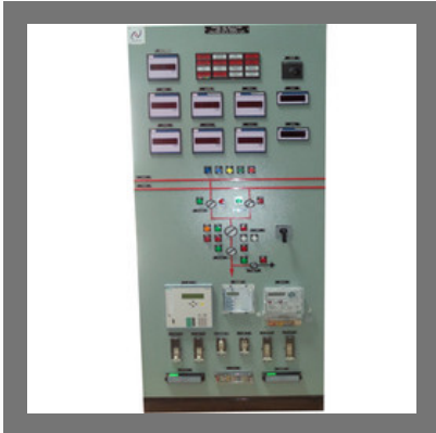
132/220 kV Line or Transformer Control and Relay Panel
